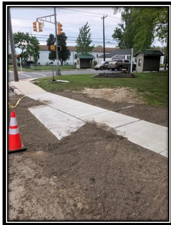
Figure: 3 – Installation of concrete sidewalk and driveway apron along the westbound lane of East Main Street approaching the intersection with Rt. 9
