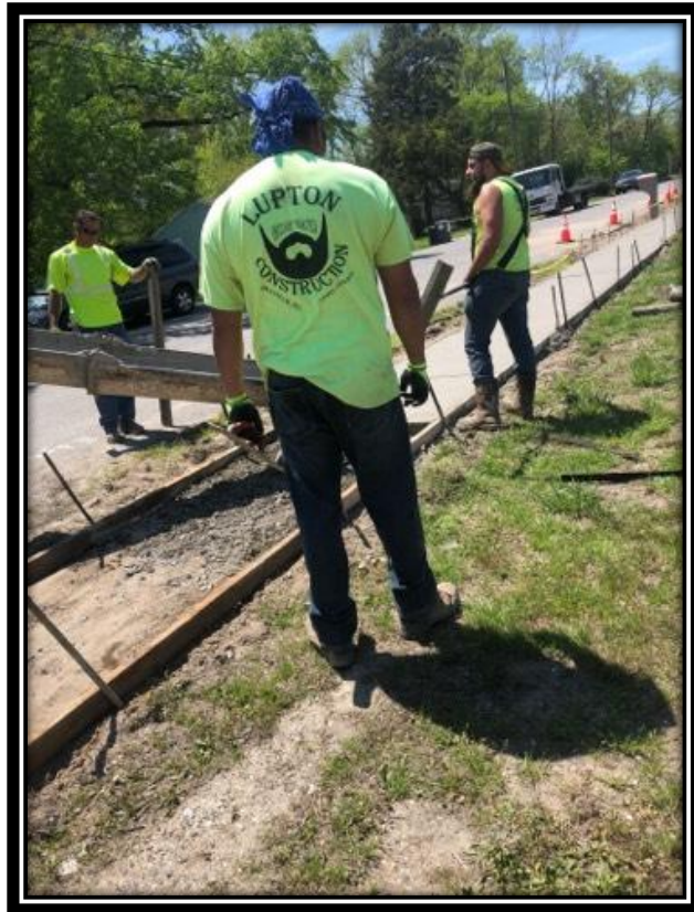
Figure: 1 – Installation of concrete sidewalk along the westbound lane of East Main Street between Rt. 9 and the historic Whitesboro School
