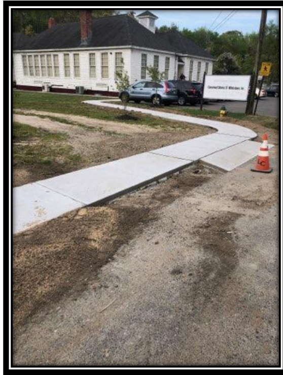
Figure: 2 – Installation of concrete sidewalk and driveway apron along the westbound lane of East Main Street approaching the historic Whitesboro School
