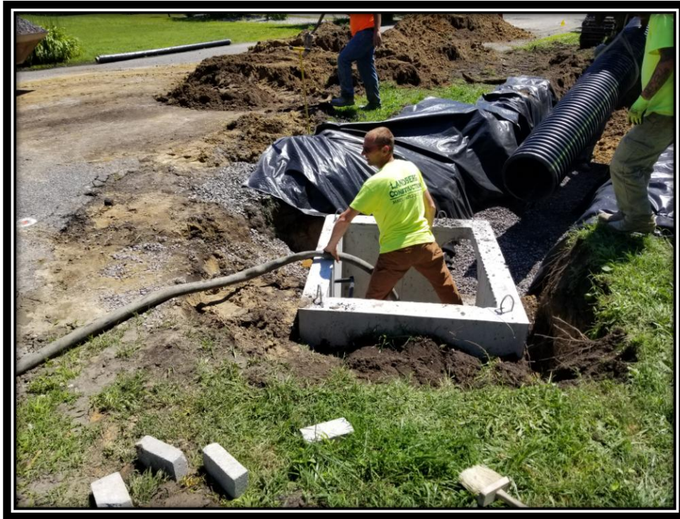
Figure: 2 – Installation of type 'C' inlet and 18" perforated corrugated plastic pipe along Pennsylvania Avenue at the intersection with South 1 st Street
