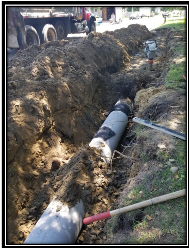
Figure: 1 – Installation of 15” reinforced concrete pipe along Pershing Avenue between New Jersey Avenue to Georgia Avenue
