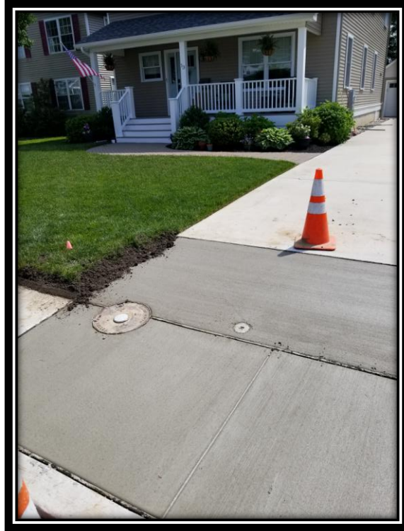
Figure: 2 – Installation of concrete driveway apron on West Atlantic Avenue along the westbound lane between South Main Street and South Boyd Street
