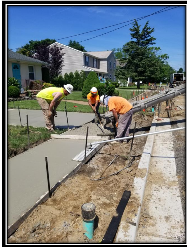
Figure: 1 – Installation of concrete sidewalk and concrete driveway apron on West Atlantic Avenue along the eastbound lane between Front Street and South Boyd Street
