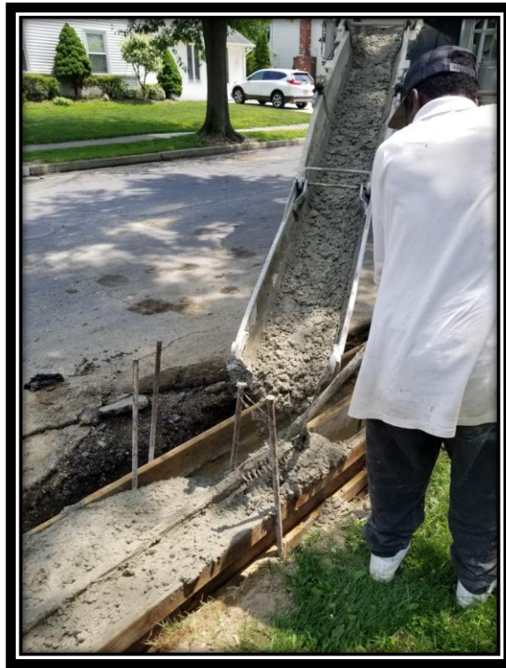
Figure: 2 – Installation of concrete curb and gutter on West Atlantic Avenue along the westbound lane between Front Street and South Boyd Street
