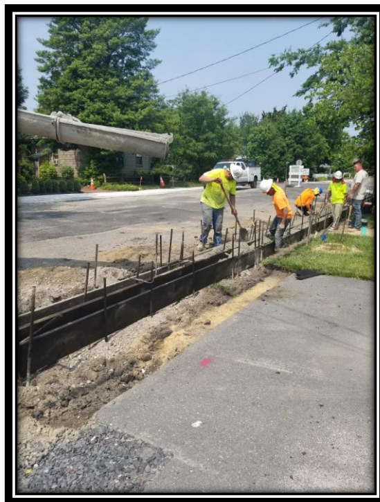
Figure: 3 – Installation of concrete curb & gutter on West Atlantic Avenue along the westbound lane between Front Street and South Boyd Street
