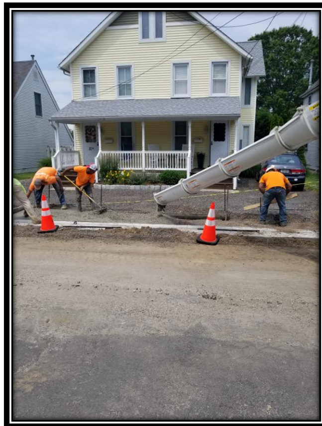
Figure: 1 – Installation of concrete sidewalk and concrete driveway apron on West Atlantic Avenue along the westbound lane between Front Street and South Boyd Street
