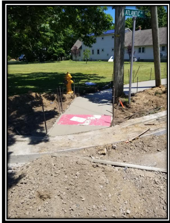
Figure: 2 – Installation of ADA ramp at the intersection of West Atlantic Avenue and South Boyd Street along the westbound lane
